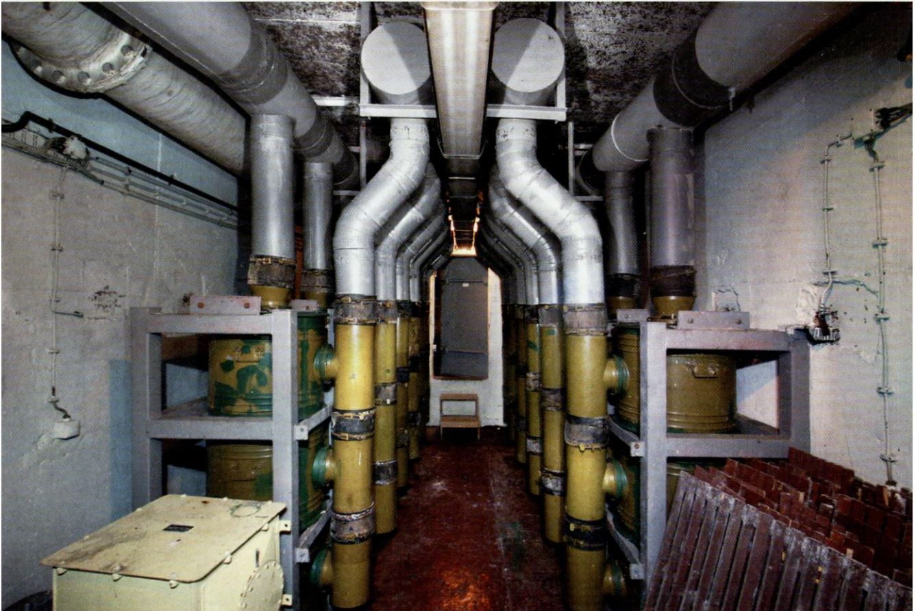
Russian made air filters in the former Volksmarine command bunker at Tessin in Germany. Photo Nick Catford
